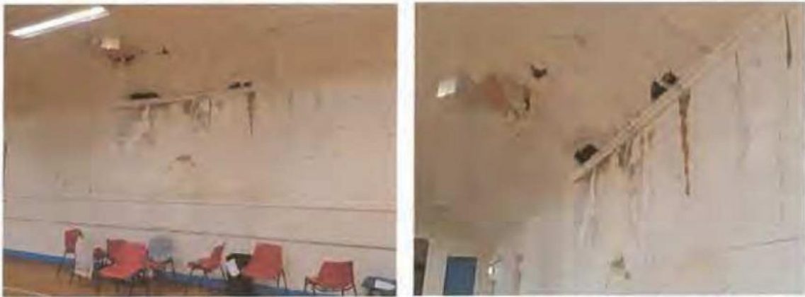
Main Hall - Ceiling and wall damage from water ingress through roof leak.
