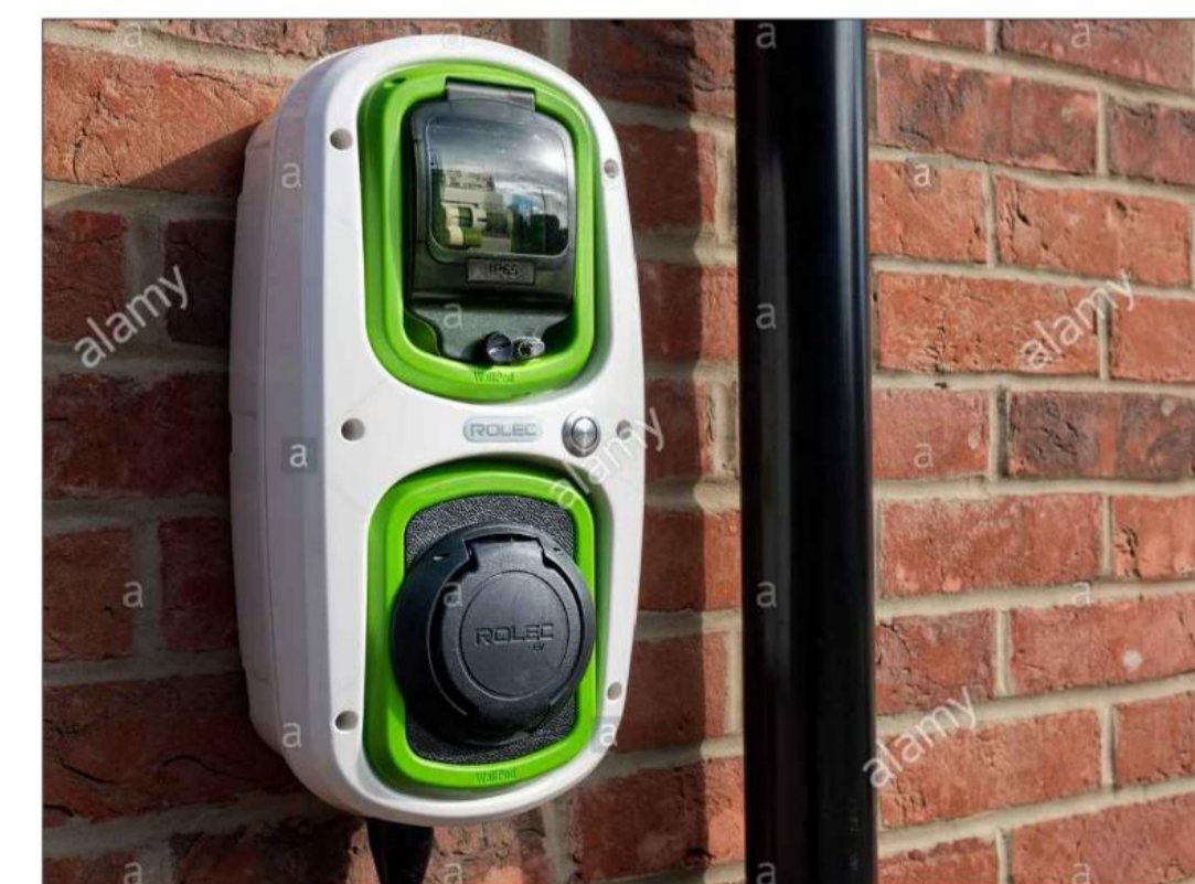
PHOTO - CHARGING POINT
