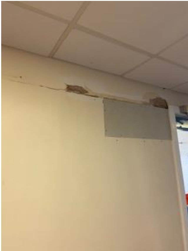
Damage to Walls/Flooring
