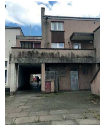
Eskdail Street - Existing buildings in poor condition and forbidding routes.
