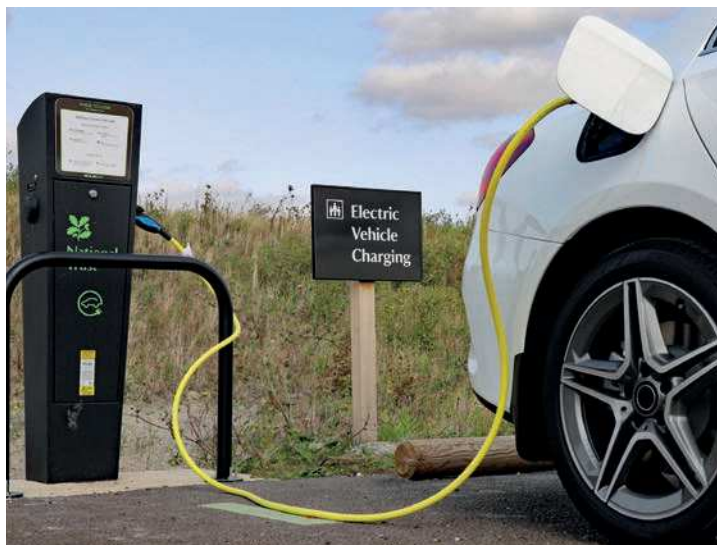
Electric Car Charging Points
