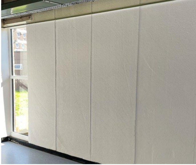
Figure 1: Images of RAAC panels – not Midlothian
